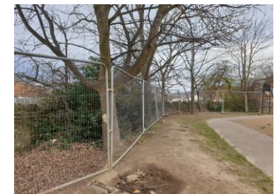
Fence requires improvement
